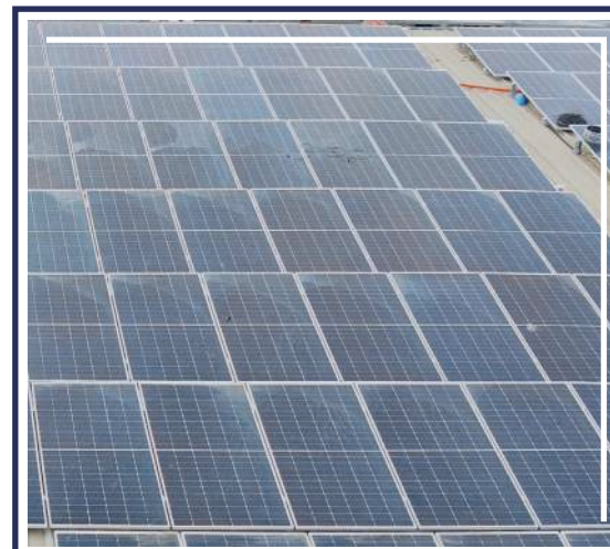
Oswal Extrusion Limited, Gandhidham Capacity - 6.02 MW
