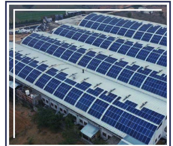
Pegma Resources, Ajmer Capacity - 600 KW
