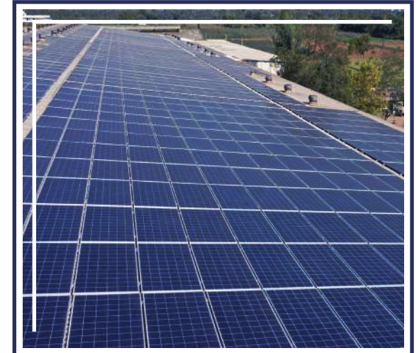
Ratnadeep Metals & Tubes, Ahmedabad Capacity - 1 MW
