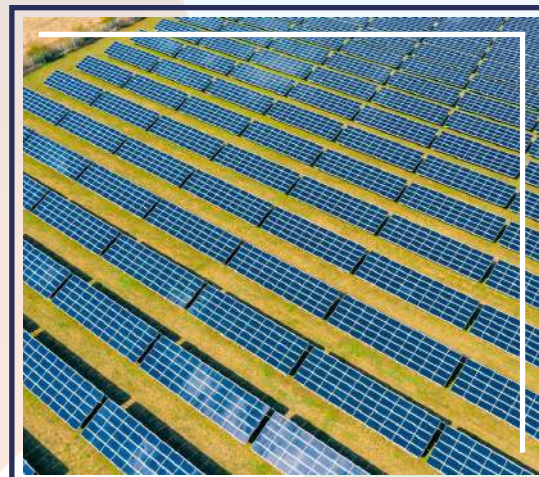
Gujarat Flotex, Ahmedabad Capacity - 6 MW
